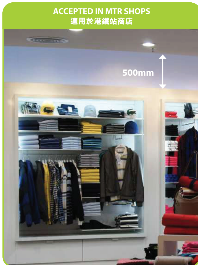
A clearance space of 500mm should be maintained below the sprinkler level as the protected area 必須在花灑頭同一水平下預留有500毫米高度距離的空間
