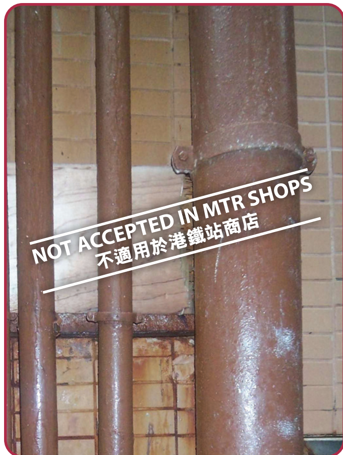
General water pipes without marking (not accepted in MTR station shops)
