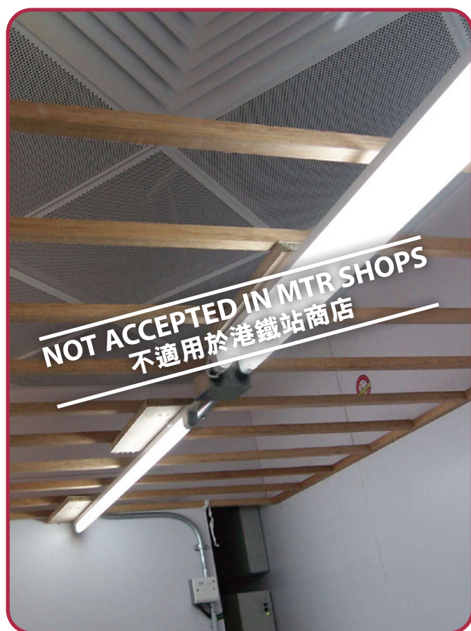
Exposed Fluorescent lighting (not applied in the visualize area) 沒有遮蔽的照明光管 (不適用於店舖的視線範圍內)
